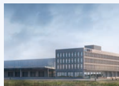
Construction of Domestic Freight Station of Freight Facility Project in the Sixth Bidding Section of China Southern Airlines Base of Beijing New Airport
