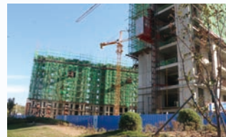
Poverty Alleviation Relocation and Integration Project in Fudong New District, Fuping County
